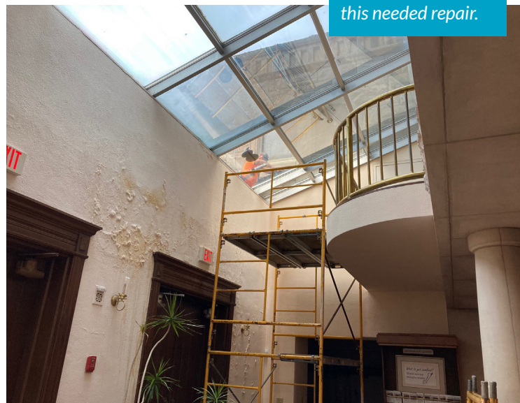
Check out the new atrium glass... now not broken! Thank you to the Second Con Foundation for this needed repair.
